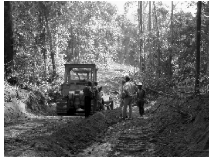
Road construction in the Wijma industrial concession, Southwest Province. Photo: Courtesy of W. Smith
